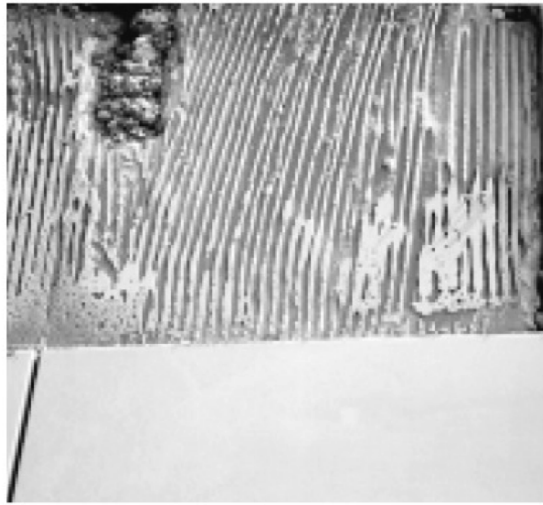
Picture 1.3 – Insufficient thin set mortar coverage. Removal of a tile reveals many voids that are present in the hardened thin set mortar. Trowel ribbons are inconsistent which will also lead to poor coverage and mortar transfer to the backs of the tiles.
