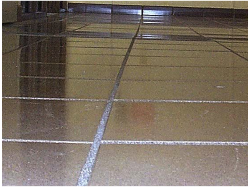
Picture 1-1 – Large format tile highlight imperfections in the substrate.
